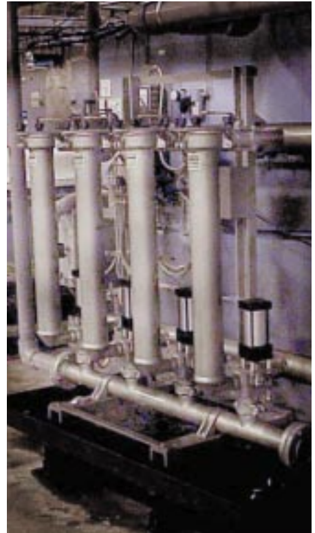
Ronningen-Petter F-Series filters were installed to help meet environmental “green” standards.
