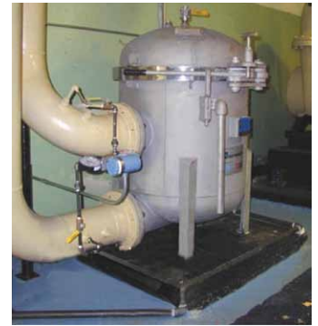
Eight bag Quick Closure vessel cooling loop, Penn Plaza, NY
