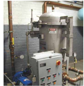
Filter Package with Pump and Control Panel
