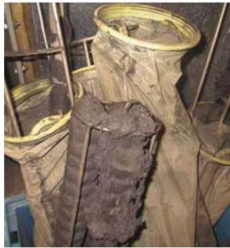
Debris removed from one Eaton filter using magnetic inserts and DURAGAF bags
