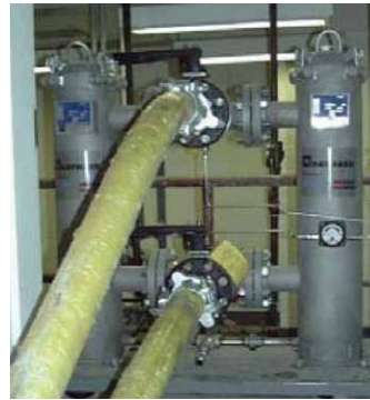
Duplex cart system on new building start-up, Times Square, NY
