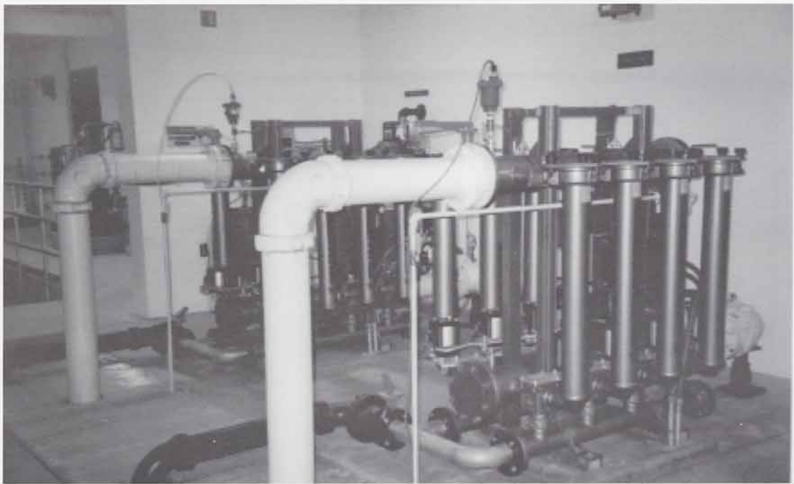
Figure 1. Ronningen-Petter F-Series tubular filters receive the incoming water from the ozone contact chamber. The pumped water leaves the ozone contact chamber at 40 to 50 psi. Prior to entering the tubular filters, the water passes through a flow control valve that adjusts the volume of water to the current ultrafiltration process needs. This volume varies depending on the number of ultrafiltration skids on line (up to four total). The water then passes through a butterfly valve, an air reducing valve, and finally a pressure reducing valve (details shown in Figure 2). This ultimately results in a pressure drop to a maximum of 30 psi to meet the ultrafiltration requirements. This pressure is not optimal for the tubular filters (recommended at 50 psi), however, operations have not been negatively impacted.
